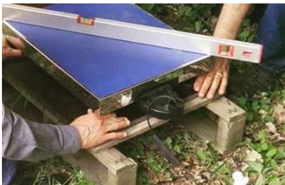
Figure 7: Outdoor weight scale and sensors installation.
