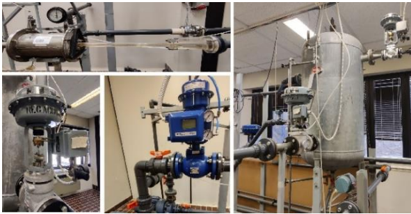
Figure 3. Experimental Plant photos
