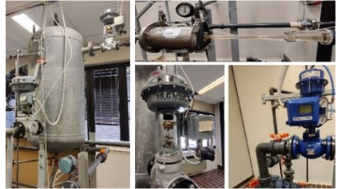
Figure 5. The experimental plant
